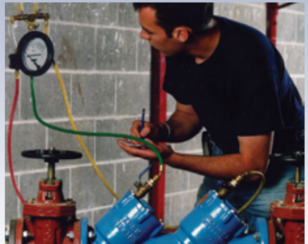
Actual testing is required by a state certified test professional. Please visit www.cewater.com/backflow for a list of certified testers.
